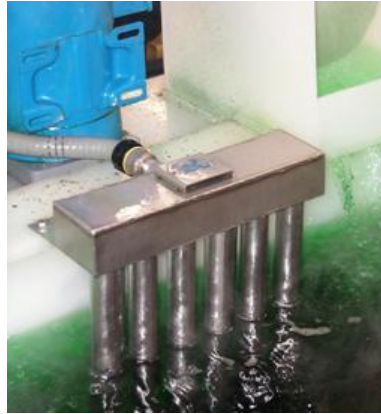
Heater with pump and bag filter
